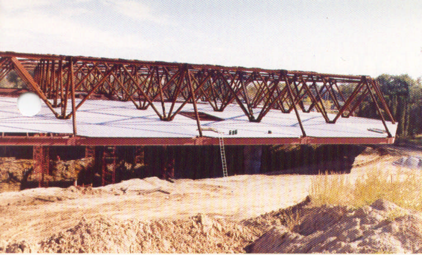
Beams and pipe trusses, held together by bolts and welded connection plates, make up the open-truss roof of the Carver-Hawkeye Sports Arena.
