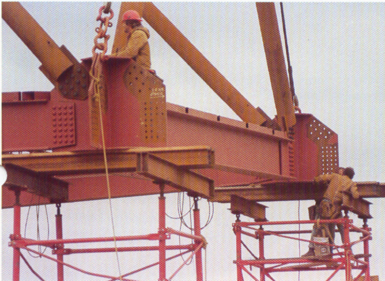
At the site, riggers fit pipe-end connection plates to plates of hub-connection assemblies, then bolt them together.
